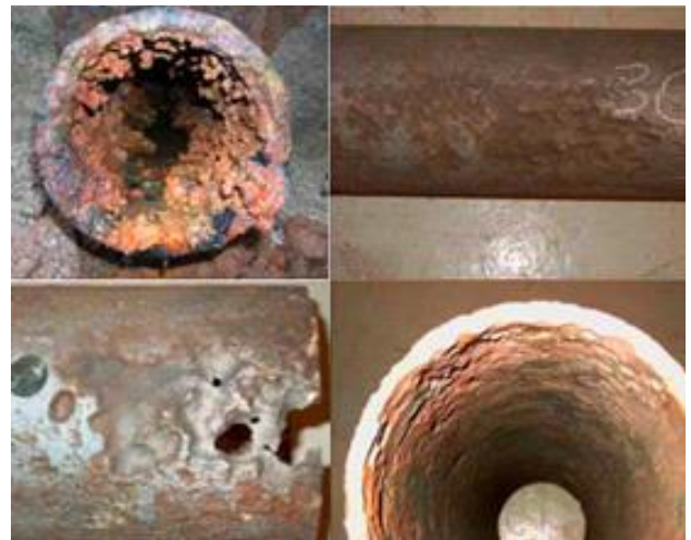
6" Cl pipe with 47% measured loss
