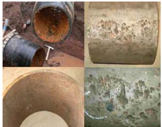
18" Cl pipe with 18.5% measured loss
