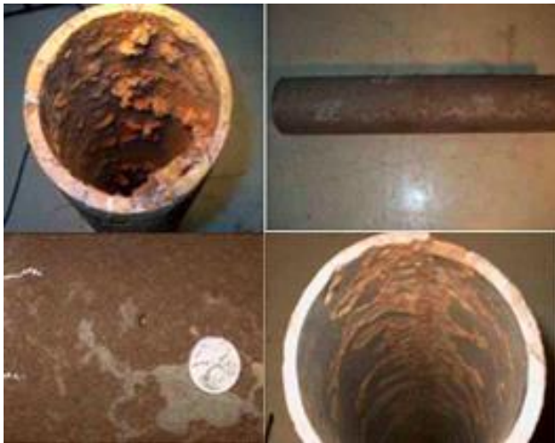
6" Cl pipe with 4.2% measured loss
